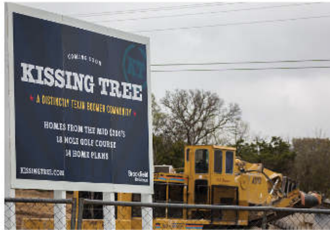
Photo by: Photo MyLife / Staff Photographer Construction site for Kissing Tree community, March 4
