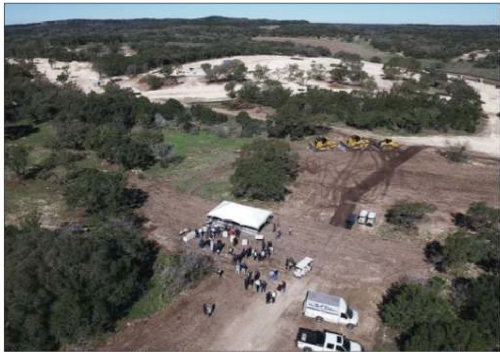
A drone captured this scene of the formal groundbreaking Feb. 25 for Kissing Tree, a subdivision for baby boomers off Hunter Road at Centerpoint. Already cleared land can clearly be seen. PHOTO COURTESY OF BROOKFIELD
